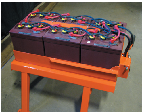
Battery Tray complete with Batteries & Watering System
